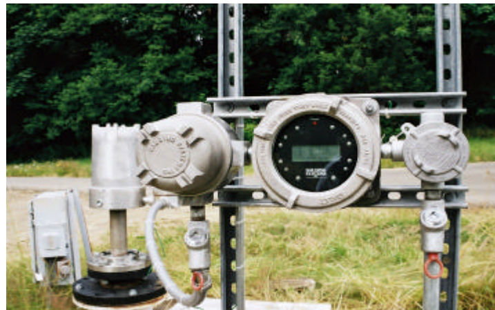
MTG in background, installed on a cut & cover (buried) tank and a TGI™ - Tank Gauge Interface
